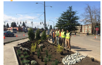
Volunteers replace asphalt with plantings along Division Ave and Sprague Ave to compliment the City's adjacent new rain garden
